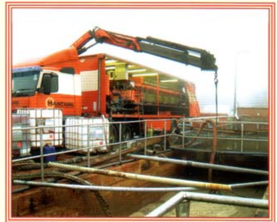
Submersible mixer pump & mobile lifting arm
